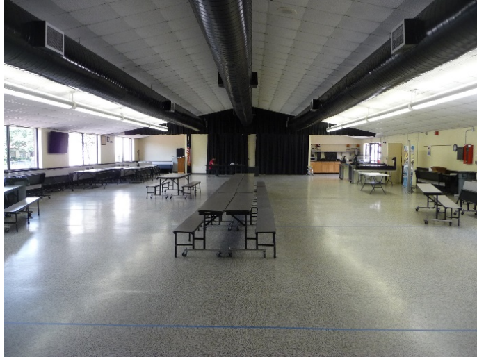
Figure 1. Interior view of cafeteria shows ventilation duct at center with space conditioning supply ducts on each side.
