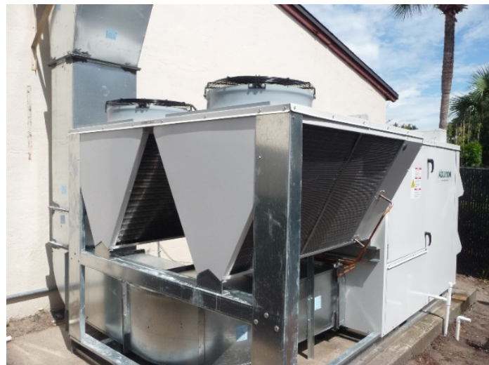
Figure 2. Addison LC 100% outside air package unit shown after installation at a high school cafeteria.
